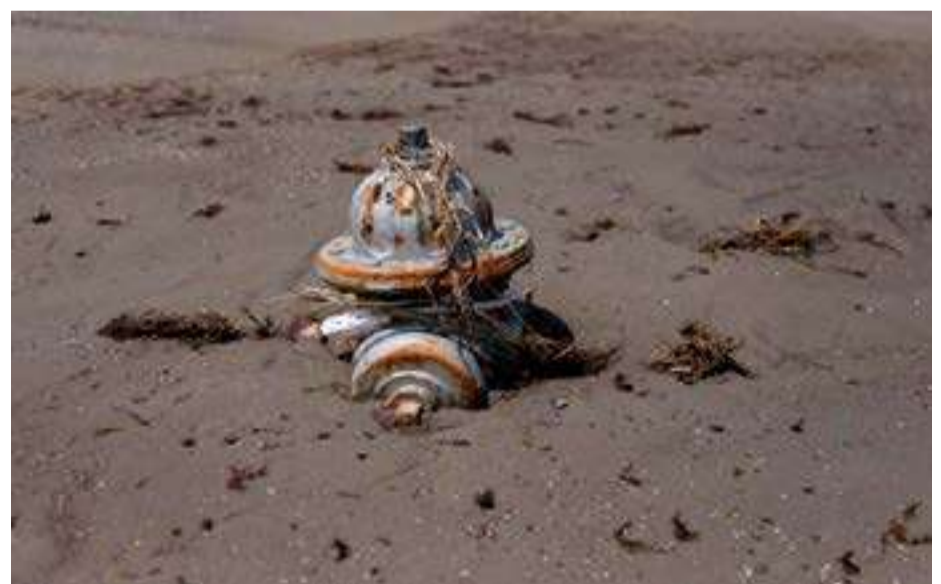
A partially buried fire hydrant can be seen days after Hurricane Ida ripped through Grand Isle, Louisiana. REUTERS/Leah Millis
