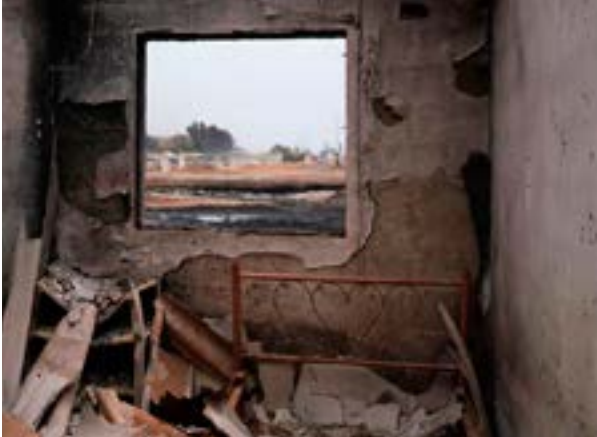
A view from inside of a destroyed house in an area of tanks that exploded near Cuba's supertanker port in Matanzas, Cuba. REUTERS/Alexandre Meneghini
