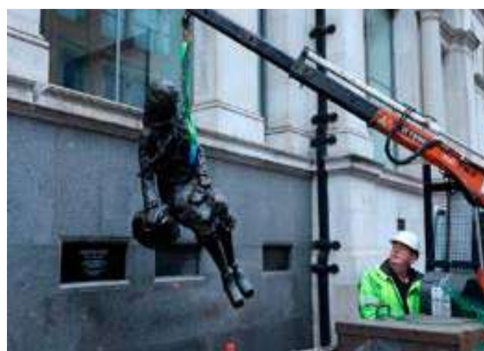
A worker uses a crane to lift a statue of Eleanor Rigby, a character immortalized in a Beatles song of the same name after it was damaged in recent cold weather in Liverpool, Britain. REUTERS/Phil Noble
